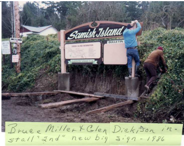
Bruce Miller and Glen Dickinson help install the second large sign in 1986.
